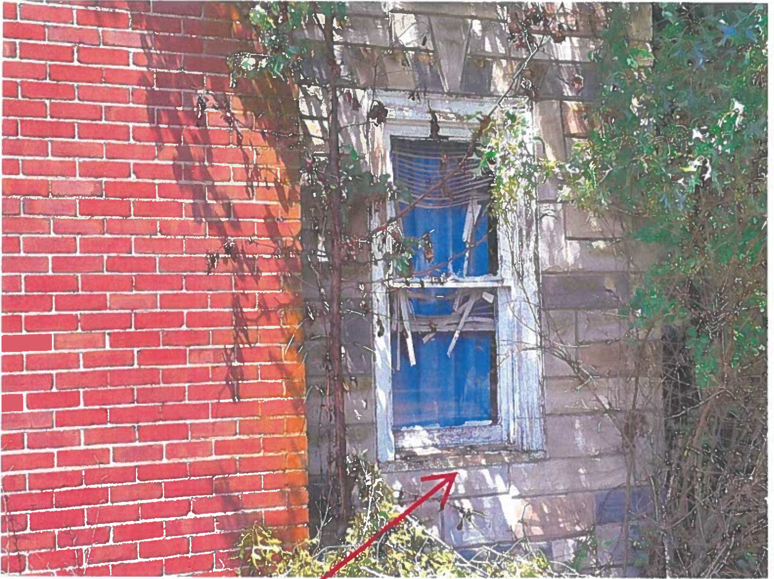
The existing windows do not show signs of broken glass, however the frame and sills are showing signs of rotting and water damage.
